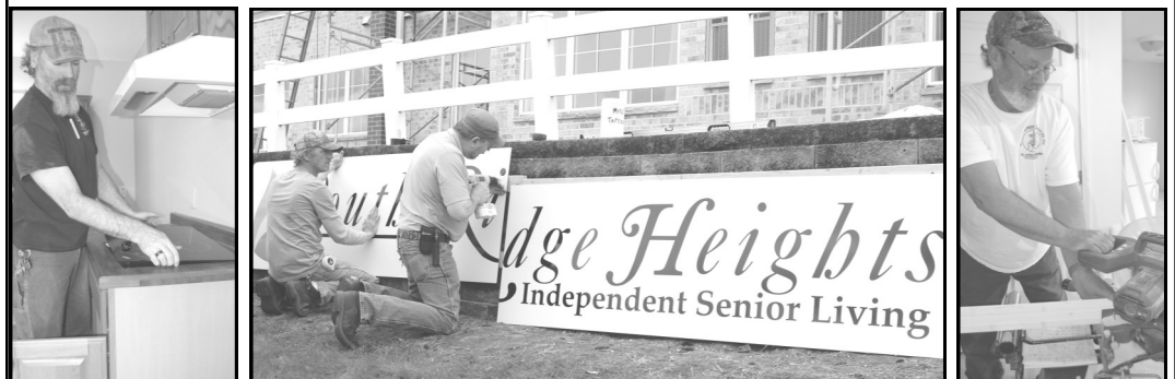
St. Luke Homes & Services maintenance men, from left, Rod Richardson, Bruce Loring, Dale Meyer and Ken Stoeber work to place finishing touches on South Ridge Heights.
