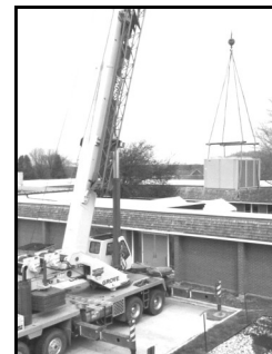
A new 50-ton air conditioning unit was installed recently in St. Luke. It replaced the original unit, installed in 1976.
